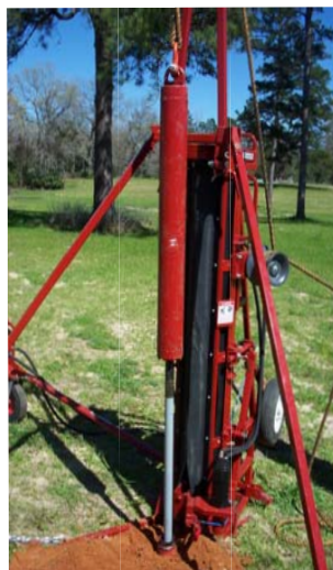
4 With the hydraulic power source at full throttle, engage cathead valve to turn cathead clockwise (looking at end of cathead). Pull rope to slowly raise hammer to connect to drill rod.
