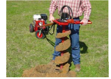
8 When hole is complete stop auger and pull out for clean hole.
