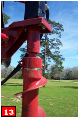
13 Lower drill head to connect drive cap to hollow stem auger. Proceed with drilling. Repeat from step 3 as necessary.
